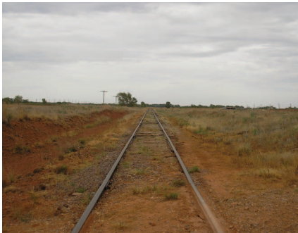
Exhibit 7: Example of Excepted Track near Sayre, OK in Need of Repair
