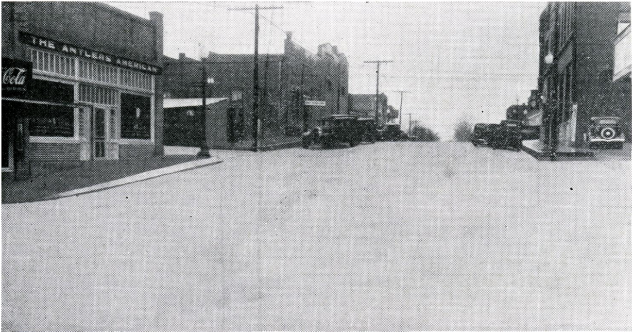
A view of downtown Antlers following a paving project. This work was part of the National Recovery Municipal project in the early 1930s.
