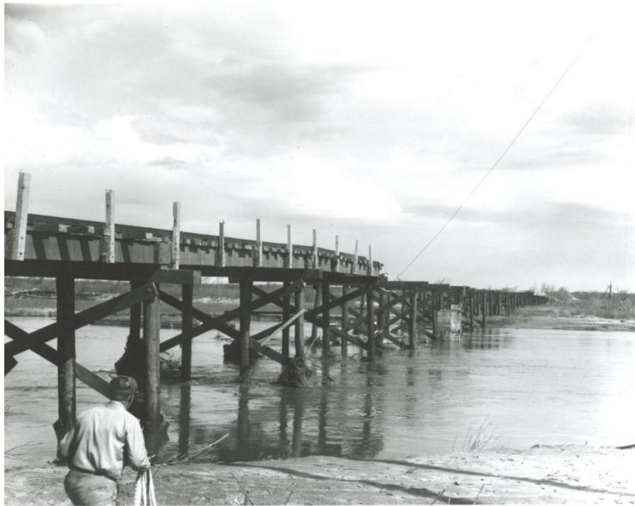
One of the many challenges for transportation is Oklahoma's weather. The 1947 Woodward Tornado is infamous for the destruction to this northwestern Oklahoma community. This view is of the damage on the SH-15A North Canadian River Bridge just after the tornado.
