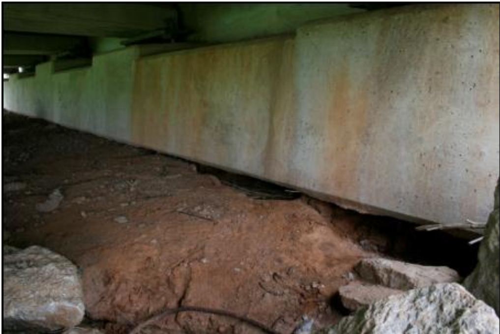
Figure 6 Erosion Under Abutment A-2, US-177 over Salt Fork
