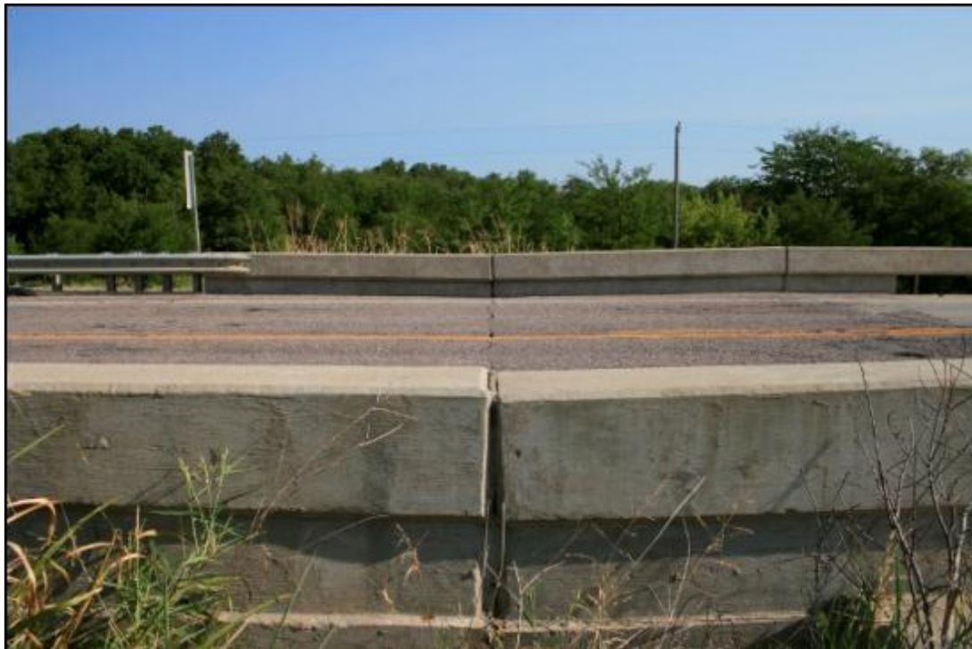
Figure 14 V-Shape Deformation of Approach No. 1
