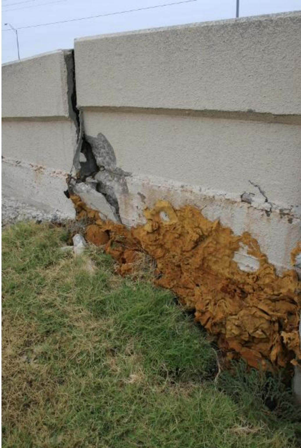
Figure 9 Maintenance and Distress Under Approach Slab
