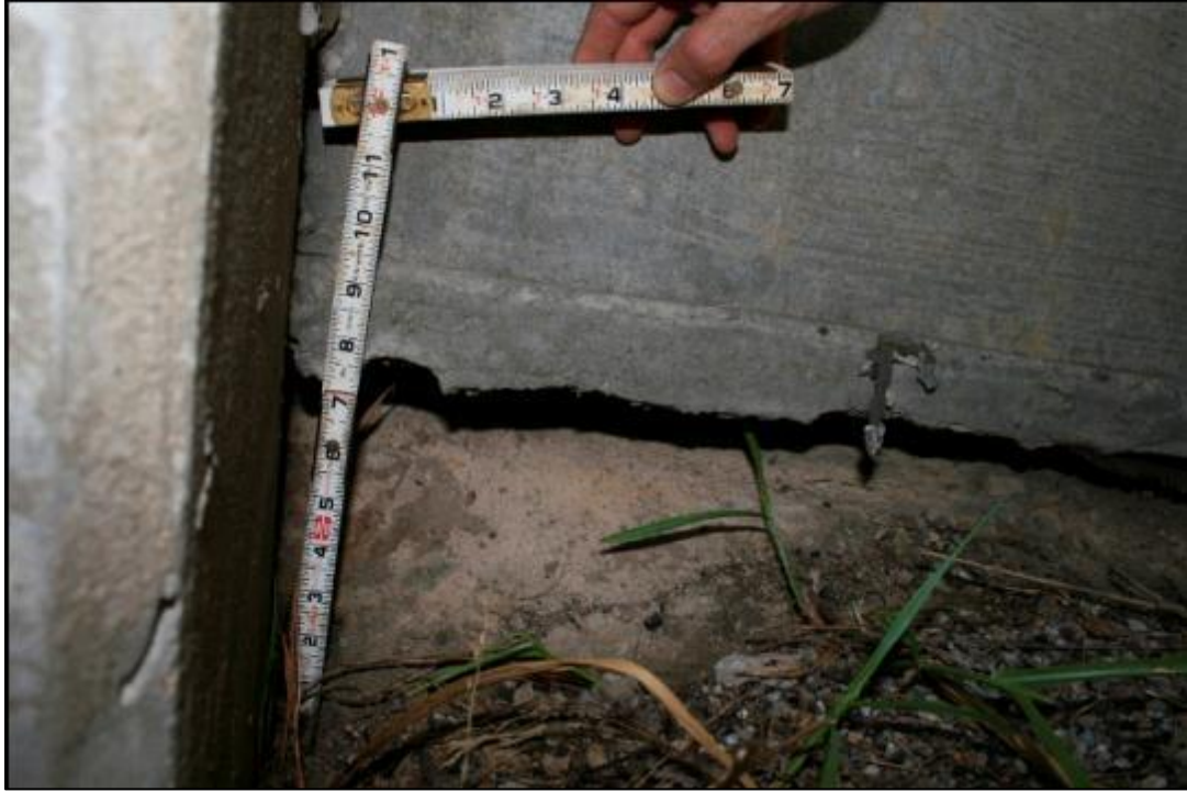
Figure 15 Void Under Approach Slab
