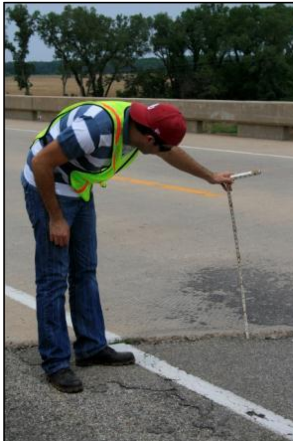
Figure 4 Karim Saadeddine Measures 2” Vertical Difference at Interface. Asphalt overlays visible.
