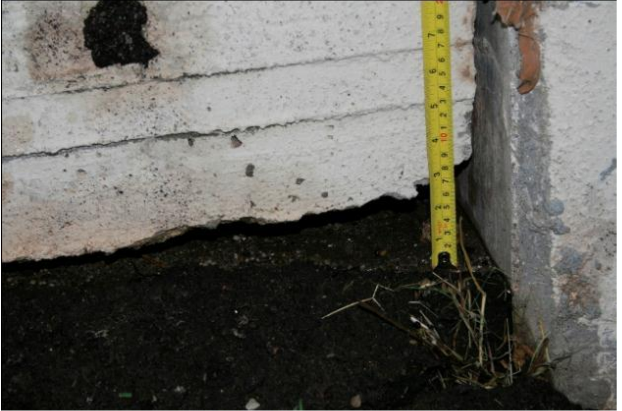
Figure 8 Void Beneath Approach Slab
