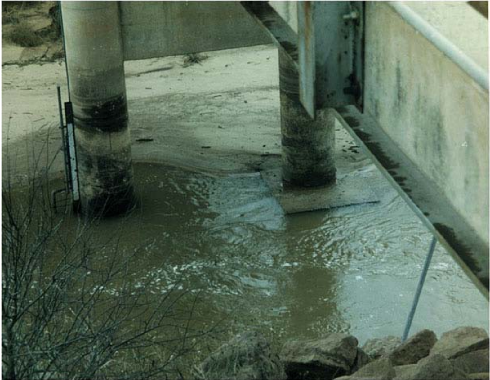
Figure 21. Picture demonstrating extent of damage to pier.
