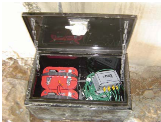
Data Acquisition Equipment in Security box under the bridge
