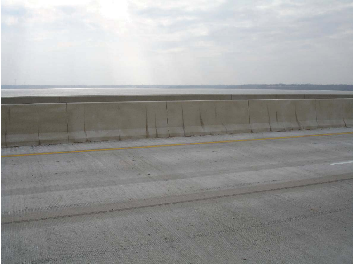
North Bridge Parapet wall showing vertical cracks – Jan. 2006
