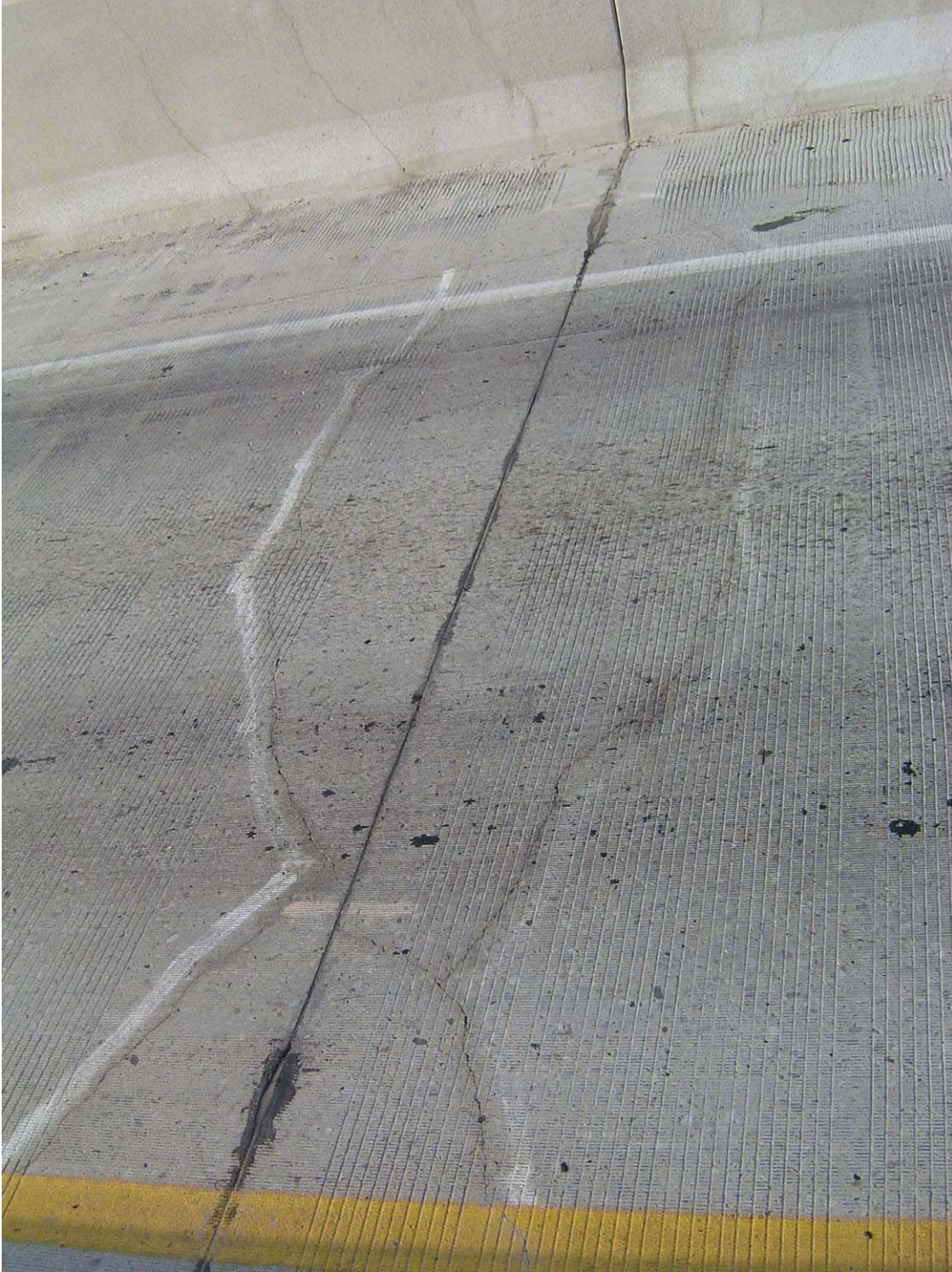
Smiley face cracks, North Bridge, north lane – July 2005
