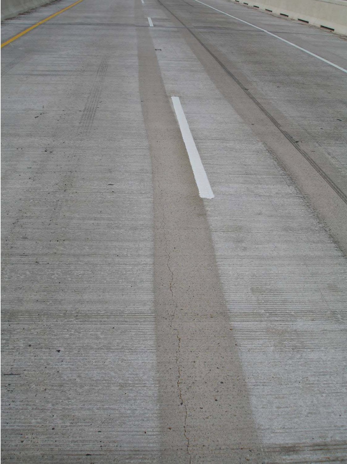
Longitudinal Cracks in North Bridge – Jan. 2006
