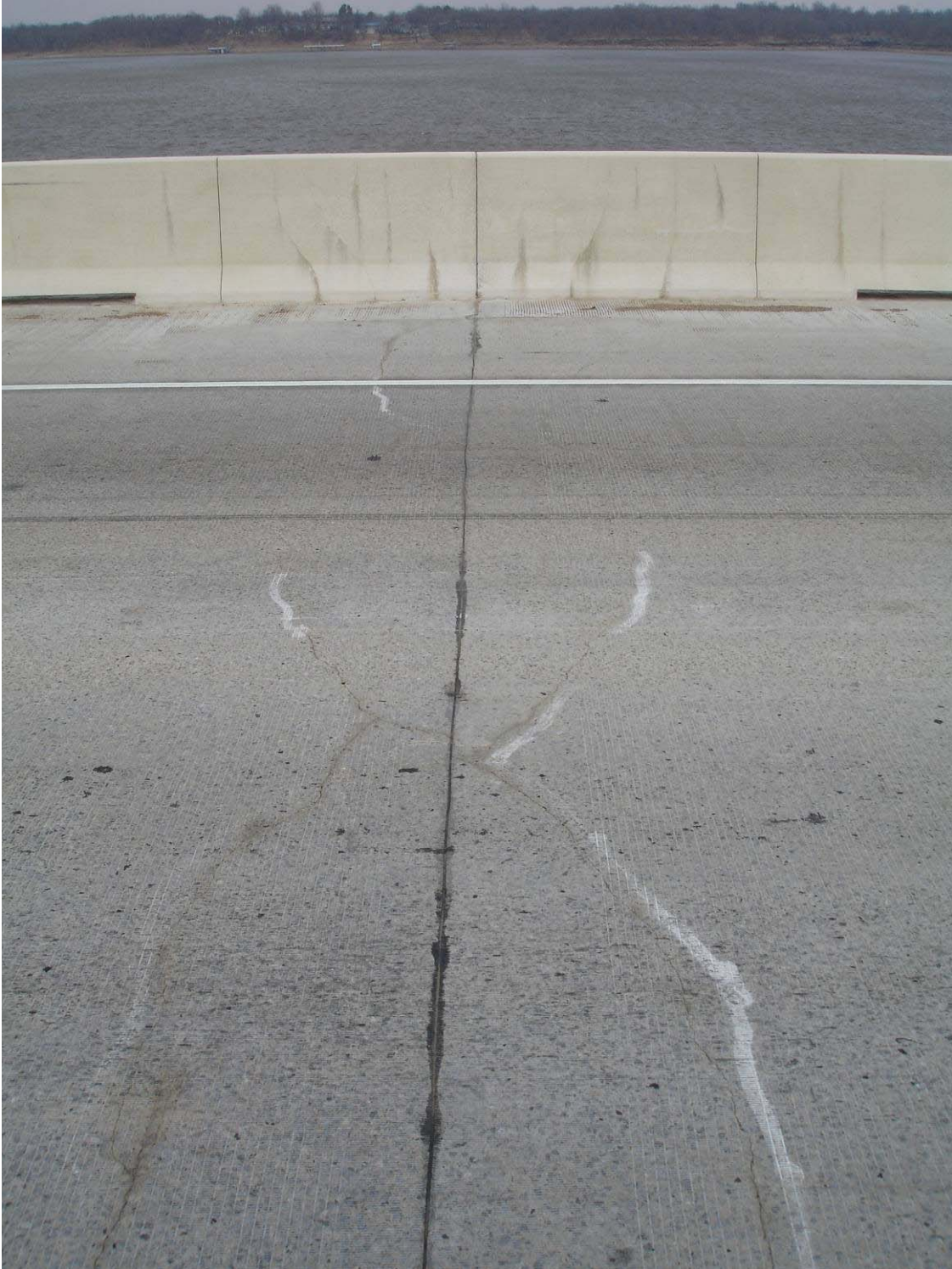
North Bridge mid-span deck "smiley face" cracks & flexure cracks in parapet – Jan. 2006
