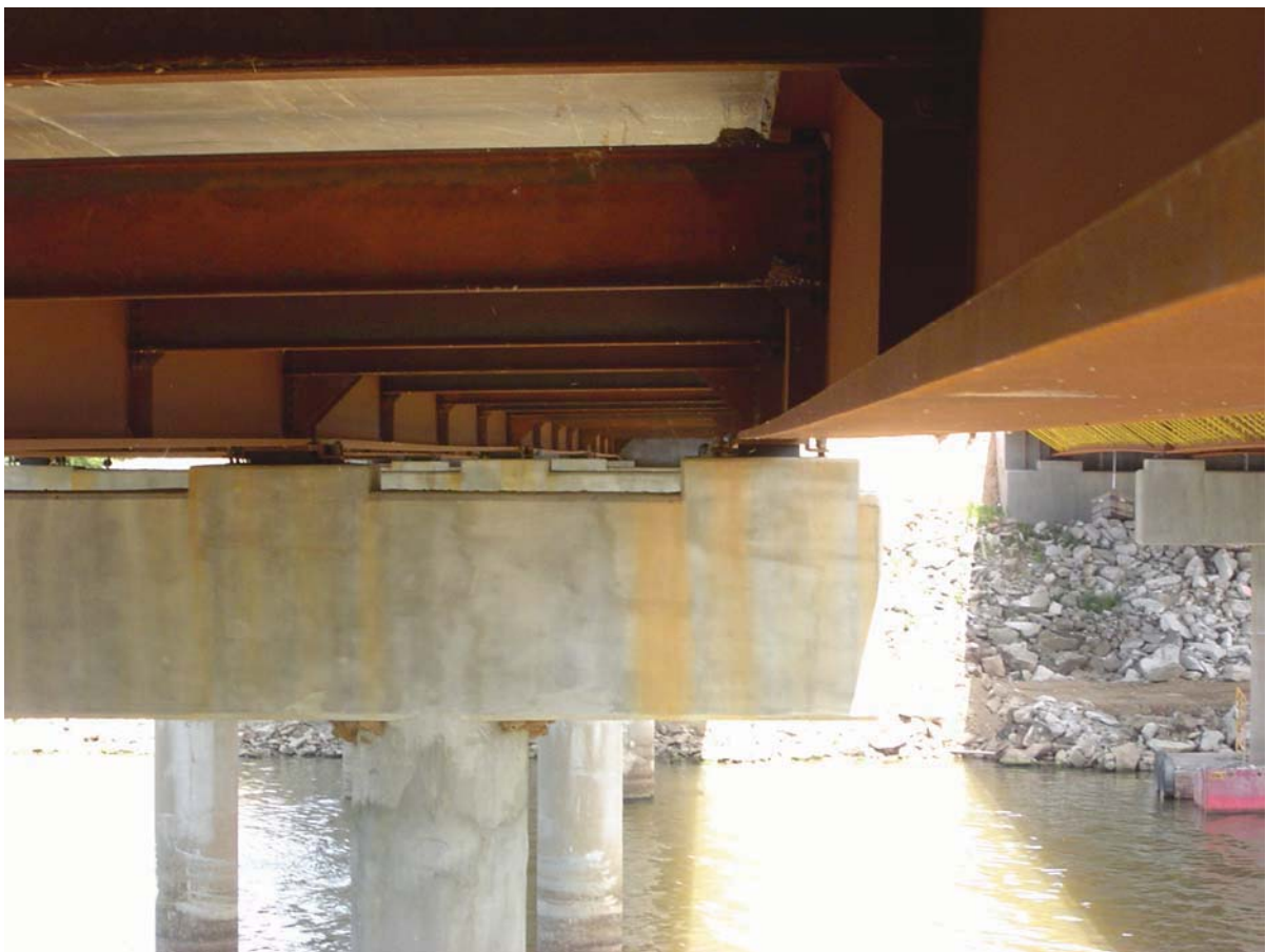
Visible deflection of North bridge girders – Note the sag in all girders
