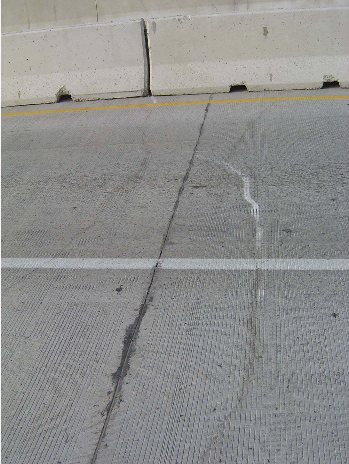
What the ODOT crews are calling "Smiley Face" cracks in deck of North Bridge at midspan North Lane - July 2005
