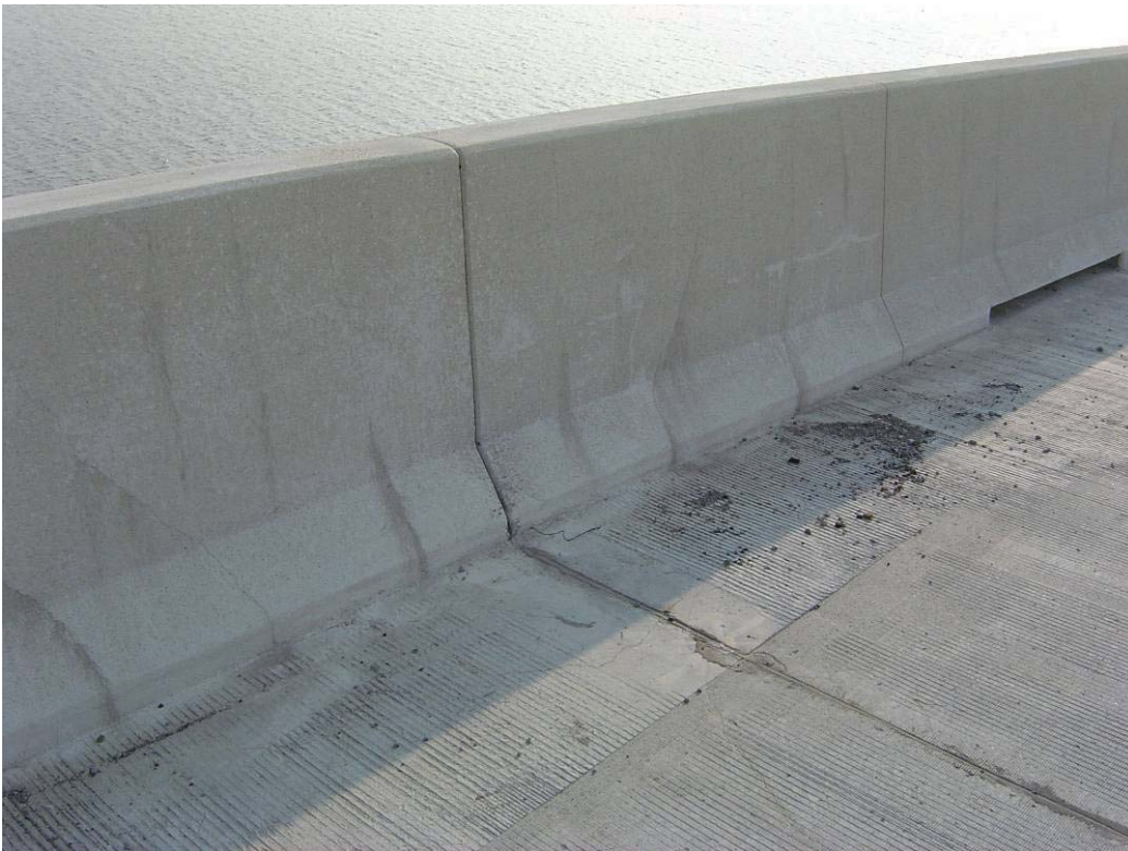
Parapet cracks in North Bridge – July 2005
