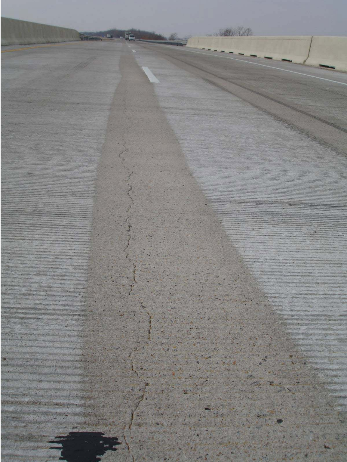
Close up of Longitudinal crack in North Bridge – Jan. 2006
