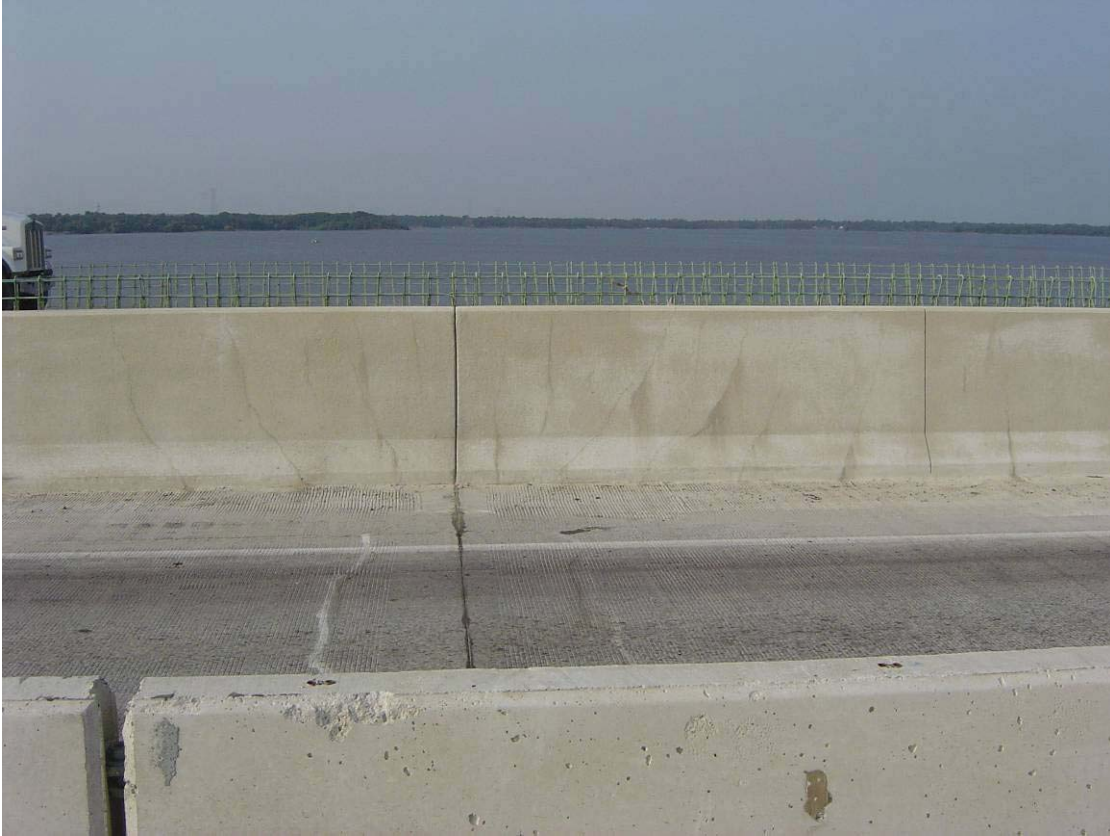
Parapet cracks in south parapet of North Bridge – July 2005
