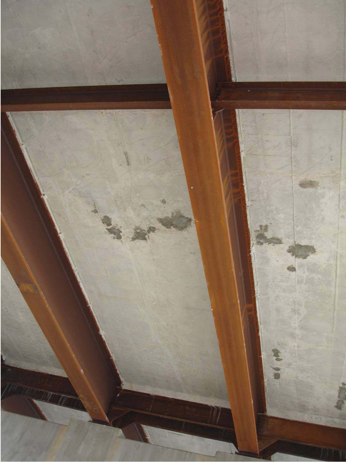
South Bridge showing water migration & cracks on bottom of deck – Jan. 2006
