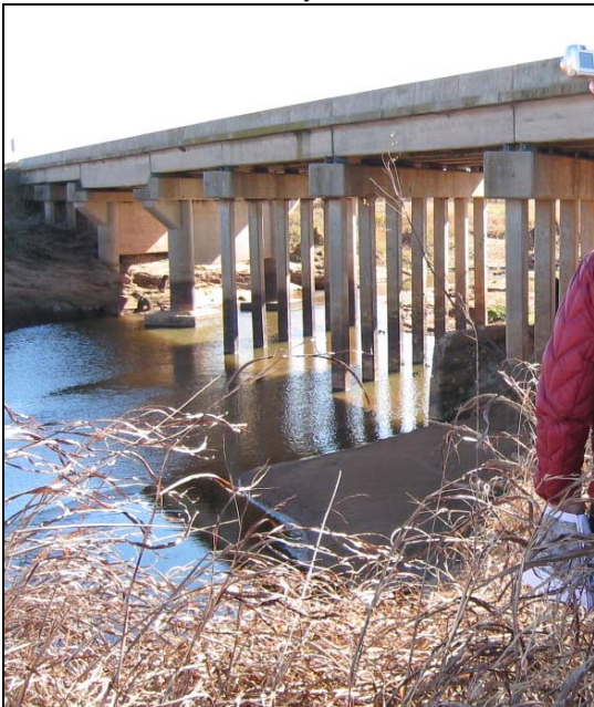
Figure B-1 Bridge scour inspection at a span bridge after a recent high-flow event, 15 November 2007.
