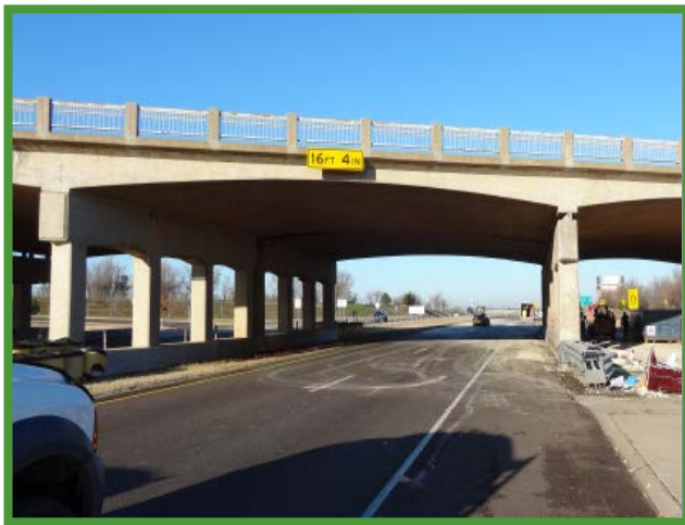
Figure 16: Substandard Truck Clearance under Anderson Road
