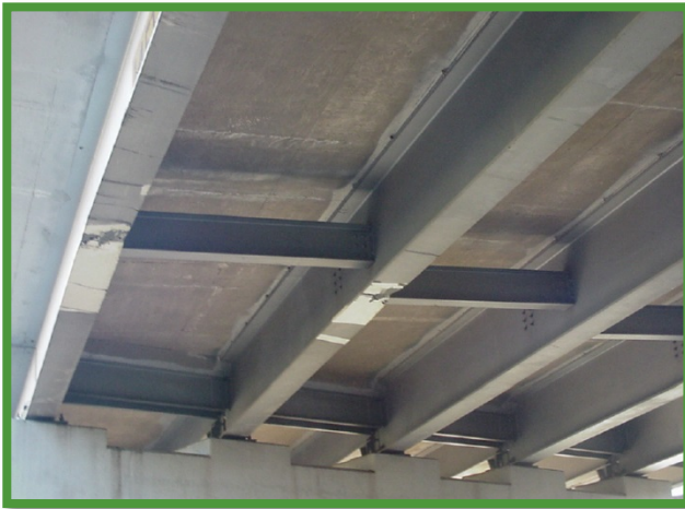
Figure 14: Anderson Road Bridge -Beam repairs needed
