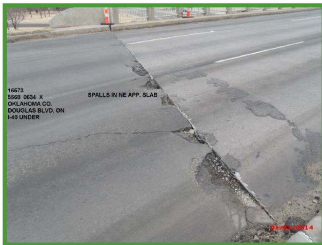
Figure 15: Douglas Boulevard Bridge - Deck repairs needed
