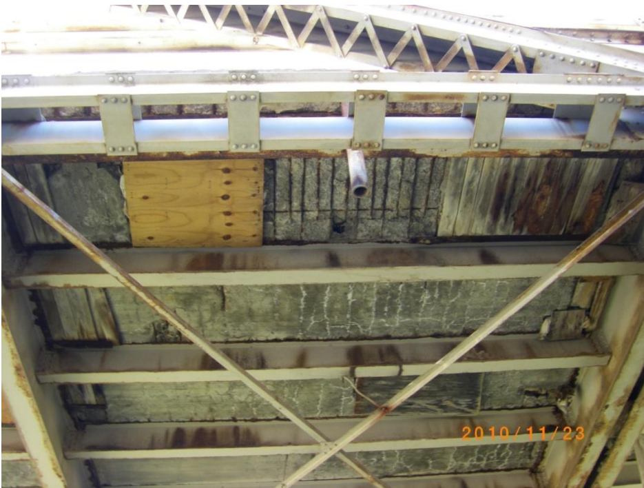
Looking underneath the westbound SH-66 bridge at Bird Creek in Rogers County, previous repairs to the deck and further deterioration are visible. Due to concerns about the load-bearing abilities of this structure, traffic is currently narrowed to one lane.
