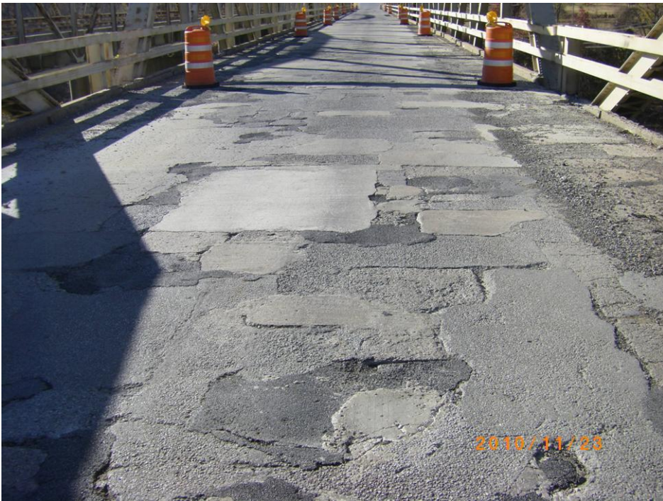
Since 2008, more than 40 emergency repairs have been made to the westbound SH-66 bridge deck over Bird Creek in Rogers County. Due to concerns about the deteriorating conditions of this bridge, it will be closed to traffic in late December.
