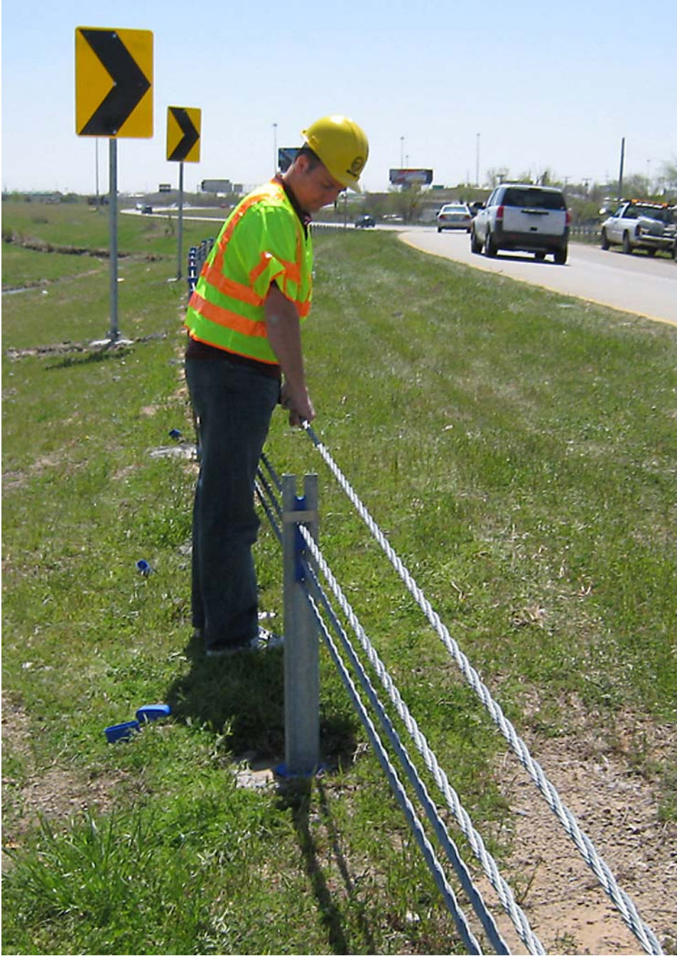
Mike Brutsche with the Oklahoma Department of Transportation's Traffic Division inspects a cable barrier at the SH-51 ramp to US-169 in Tulsa. A recent review of crash data by the Oklahoma Department of Transportation indicated a significant decrease in fatalities related to crossover accidents in areas where cable barriers have been installed.
