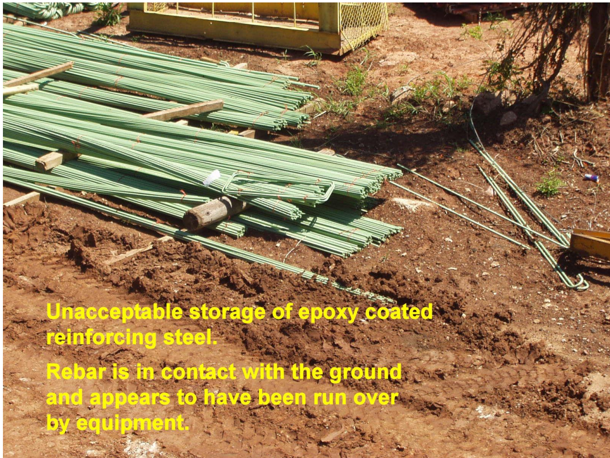
Figure 511:2. Photo. Unacceptable Storage of Epoxy Coated Steel
