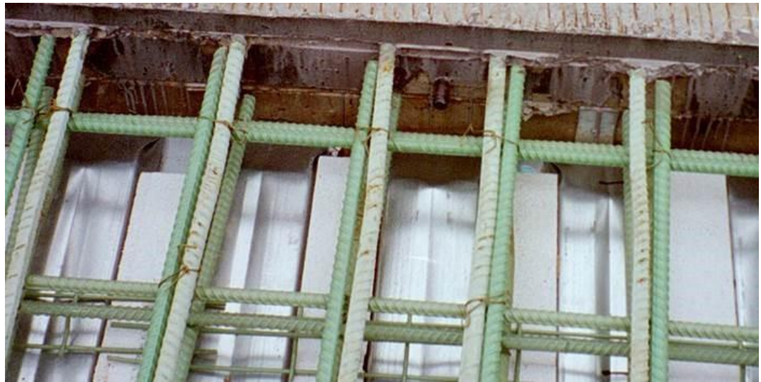
Figure 511:1. Photo. Unacceptable Exposure of Epoxy Coated Steel
