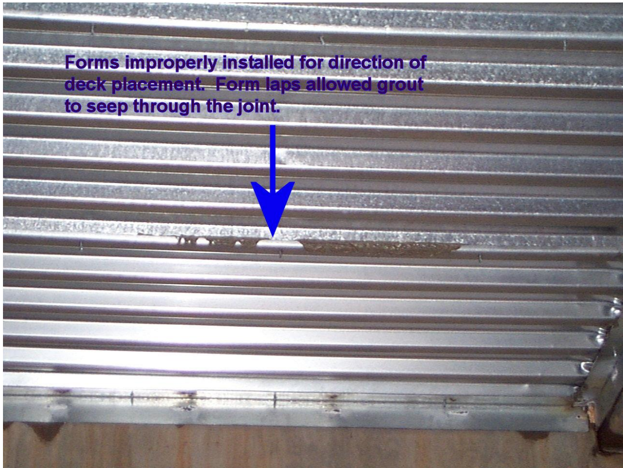
Figure 502:5. Photo. Grout Seepage Resulting from Improper Steel Form Installation
