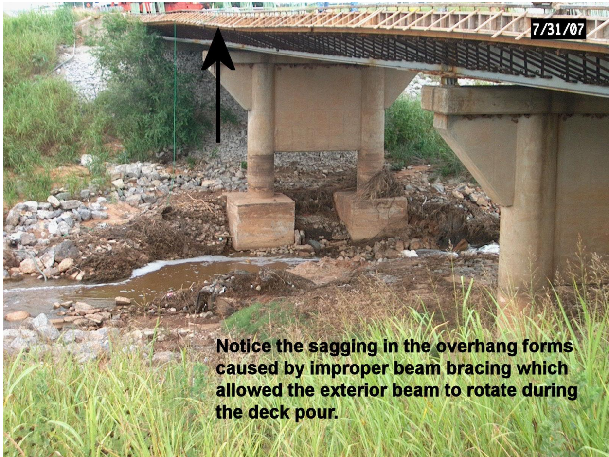
Figure 506:8. Photo. Sagging due to Inadequate Beam Bracing
