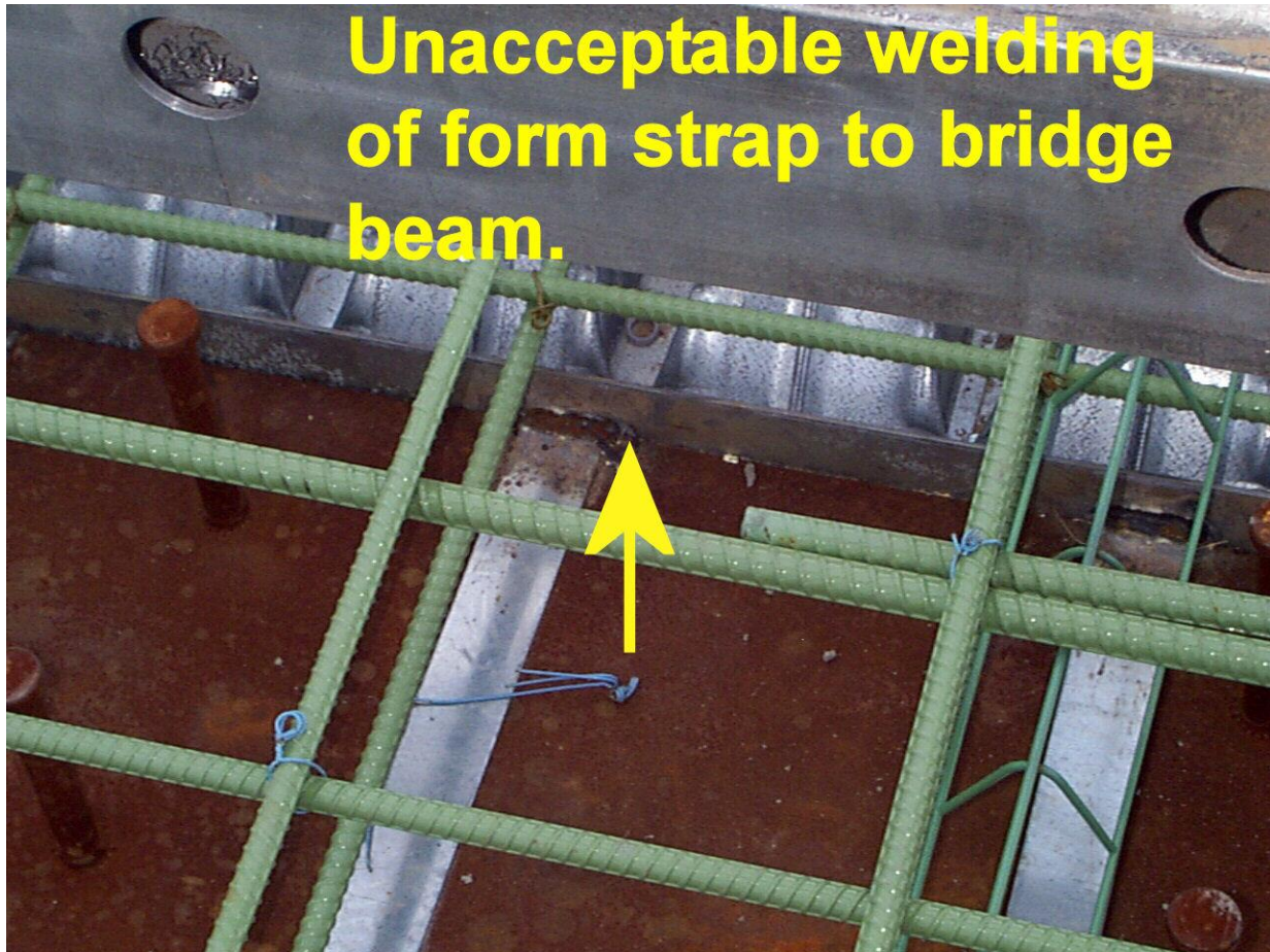
Figure 502:7. Photo. Unacceptable Welding of Form Strap to Bridge Beam
