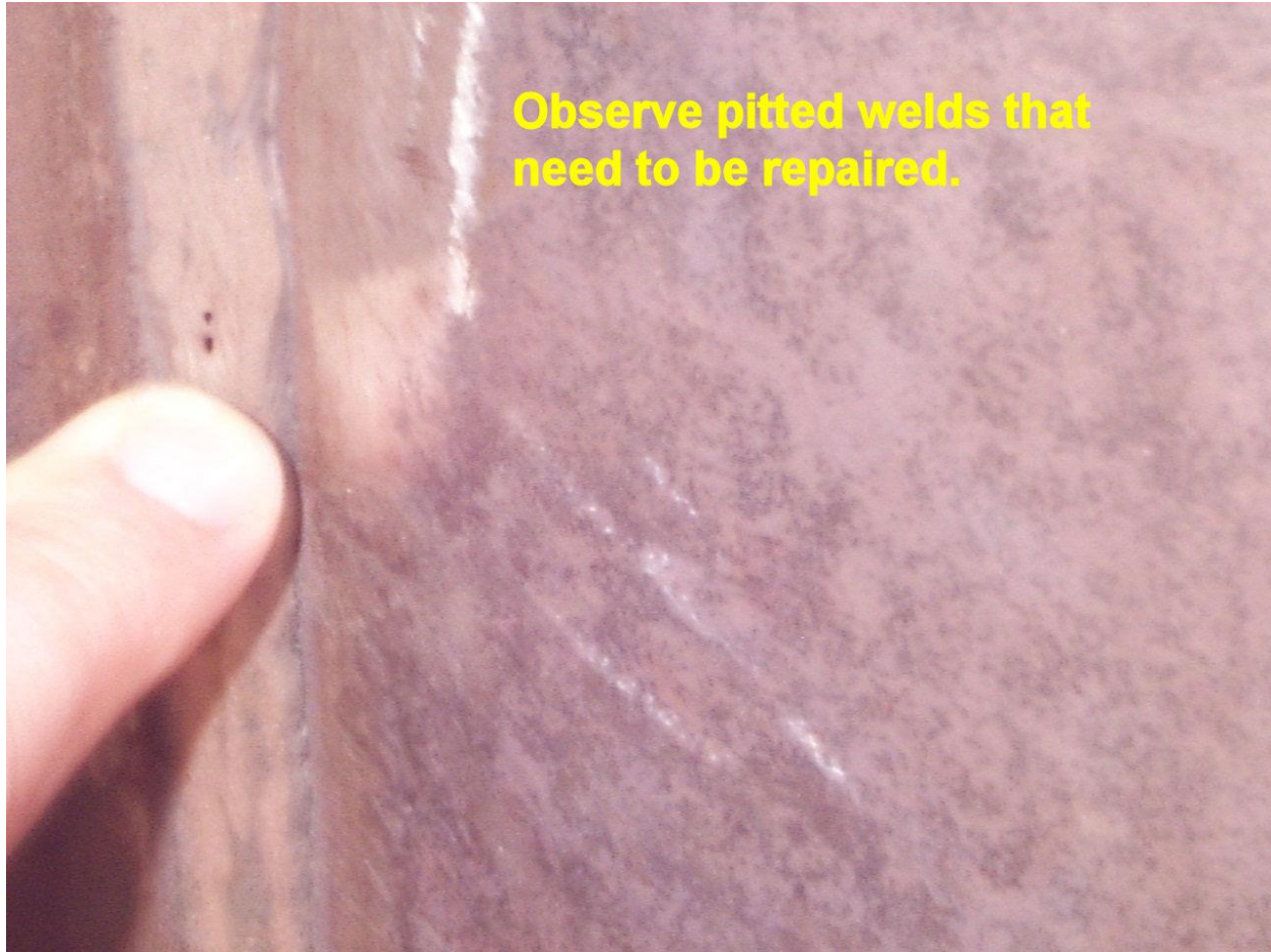
Figure 506:4. Photo. Pitted Welds in need of Repair
