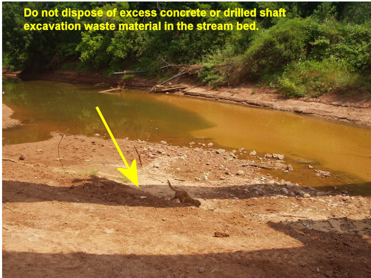
Figure 516:1. Unacceptable Disposal of Waste Materials in Stream Bed
