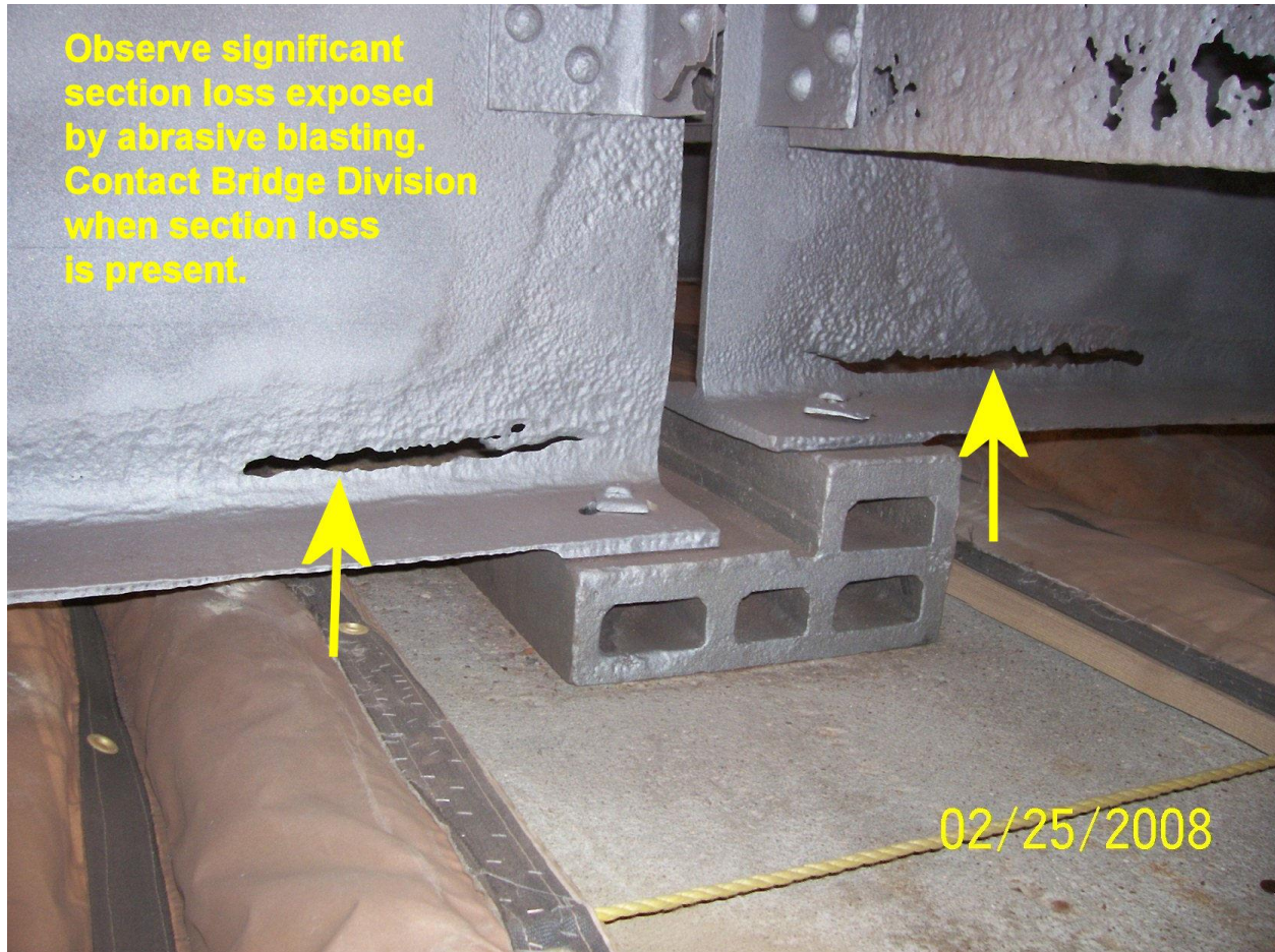
Figure 512:1. Photo. Section Loss caused by Abrasive Blasting
