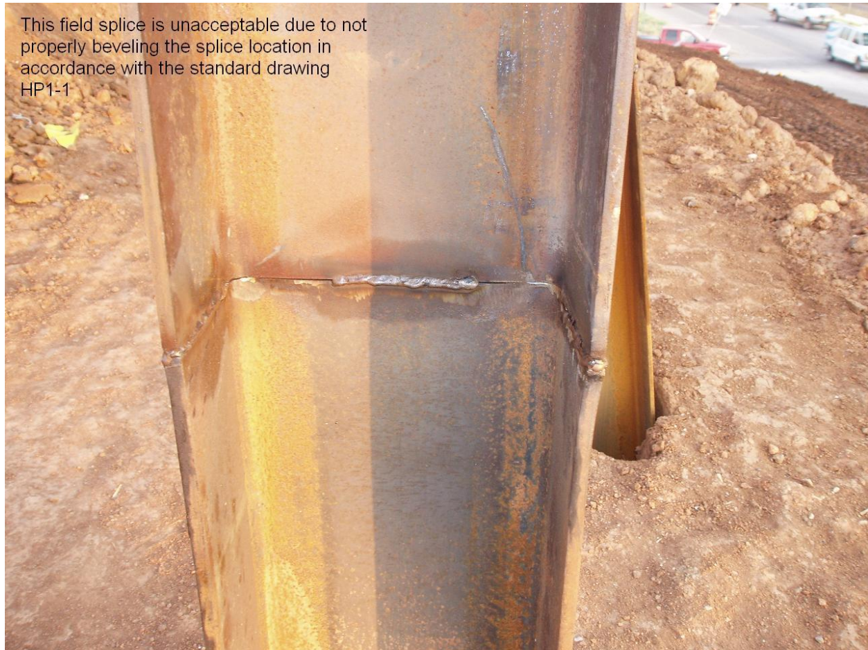
Figure 514:3. Photo. Unacceptable Field Splice
