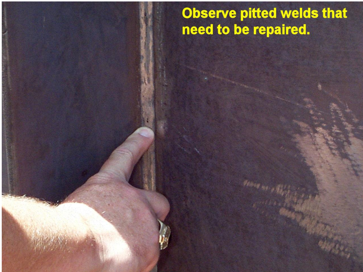
Figure 506:3. Photo. Pitted Welds in need of Repair
