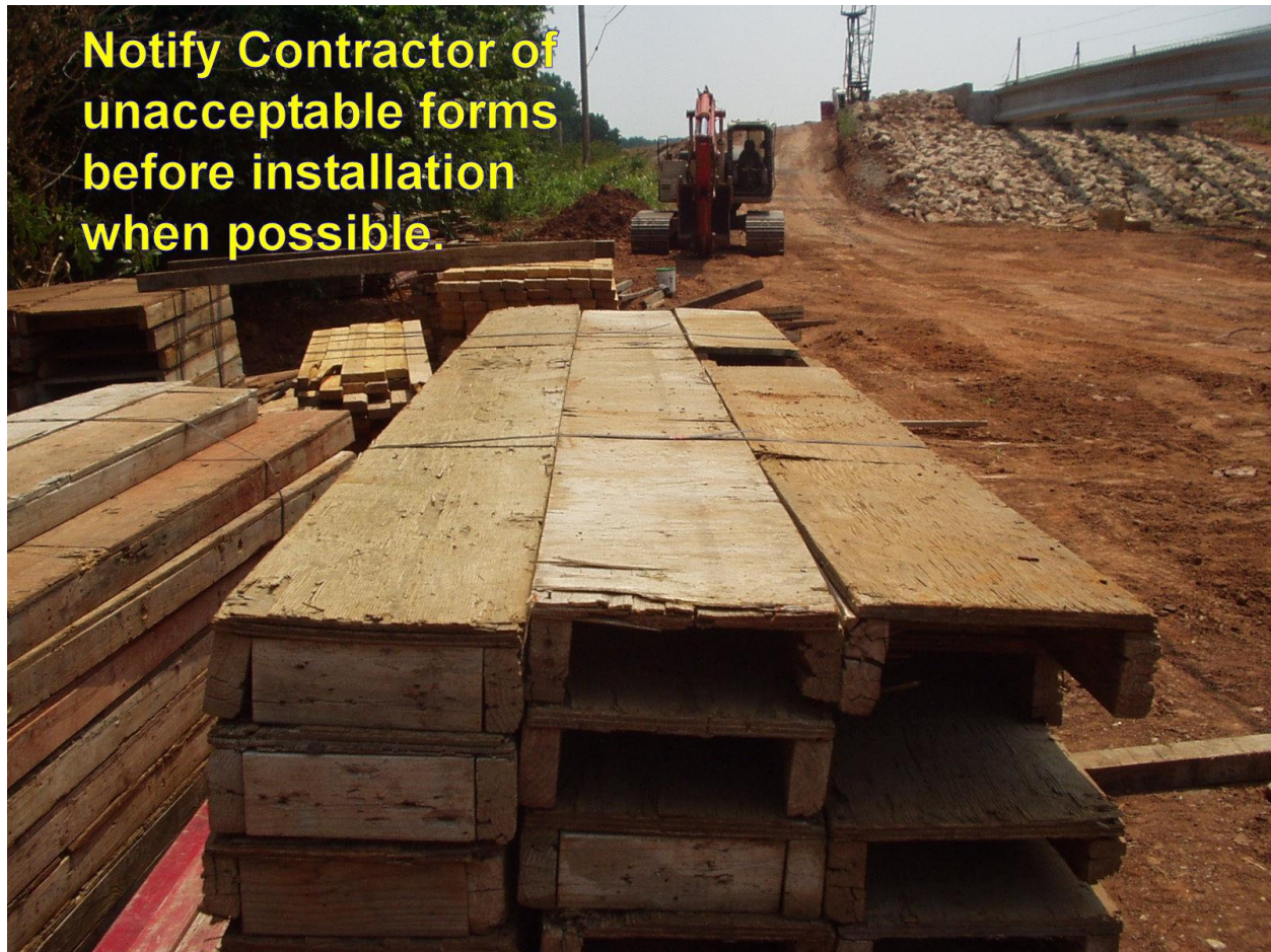
Figure 502:3. Photo. Unacceptable Forms
